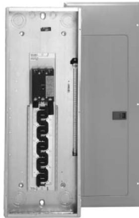
Main Circuit Breaker
